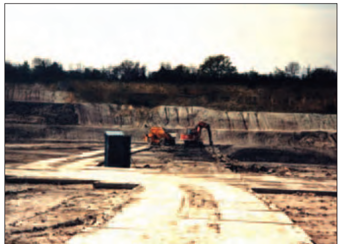
Loading dump truck by hydraulic face shovel with temporary roadways laid as an internal haul route.
